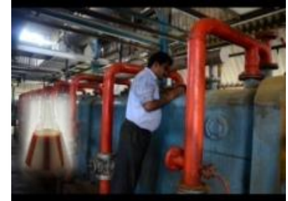
Solvent Crude Butter Extractor
