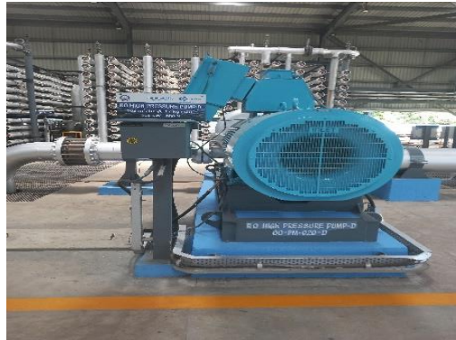
High pressure RO pump
