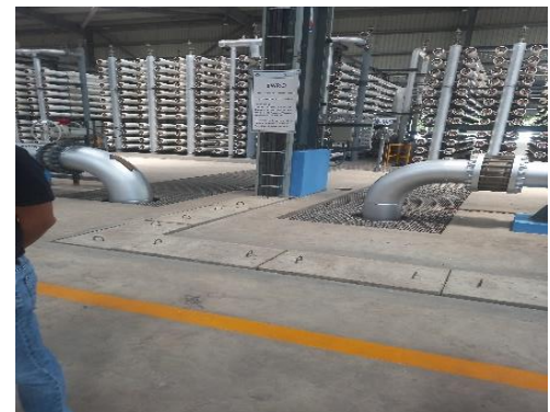
RO Filtration Section
