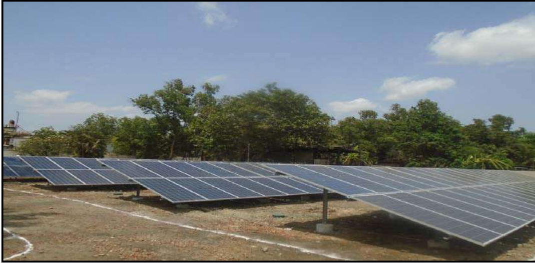
Figure 5.1 Solar power plant installed on site of TDMCCL
