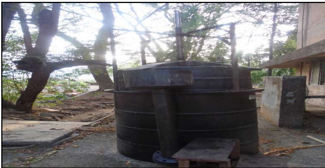
Figure 5.4 Biogas Plant on site of TDMCCL
