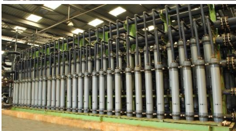
110 MLD SWRO (Desalination) Plant, Nemmeli, Chennai, India India's largest operational desalination plant till date
