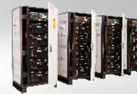
Power Backup System
